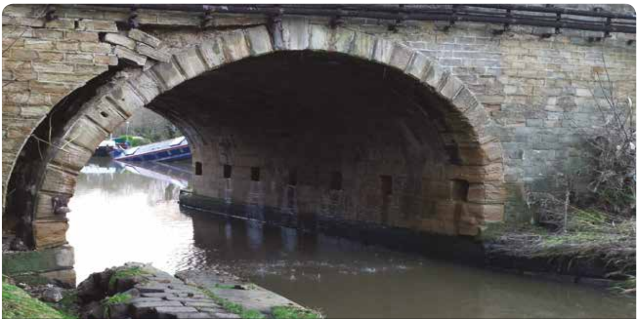
Grade II listed Elland Bridge, Calder Valley, which was seriously damaged by flood water in 2015's Storm Eva
